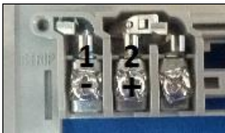
Strobe Wiring Terminals
